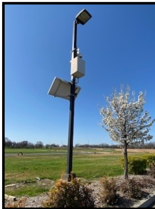
Figure 1 Plumas Lake camera set up with solar.
